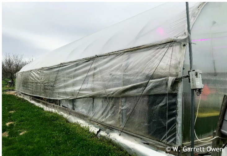
Figure 5. High tunnel where the motorized sidewall crank system failed to open. Photo by W. Garrett Owen.
